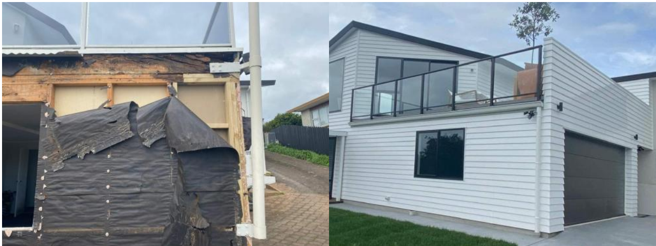
BEFORE — hidden damage found once cladding was removed
